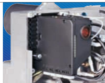
Control box fitted with ignition transformer
